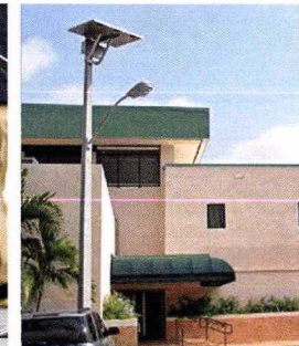
Solar Street Lighting as existing
