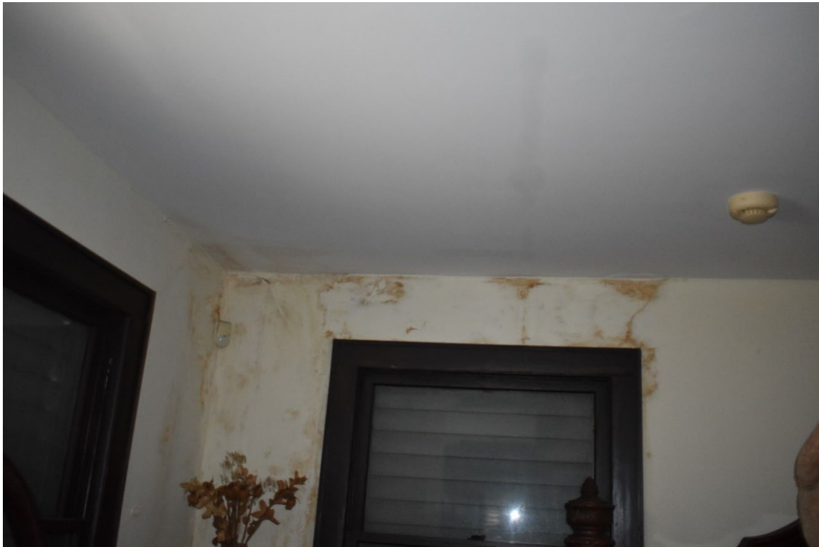
View of water damage
