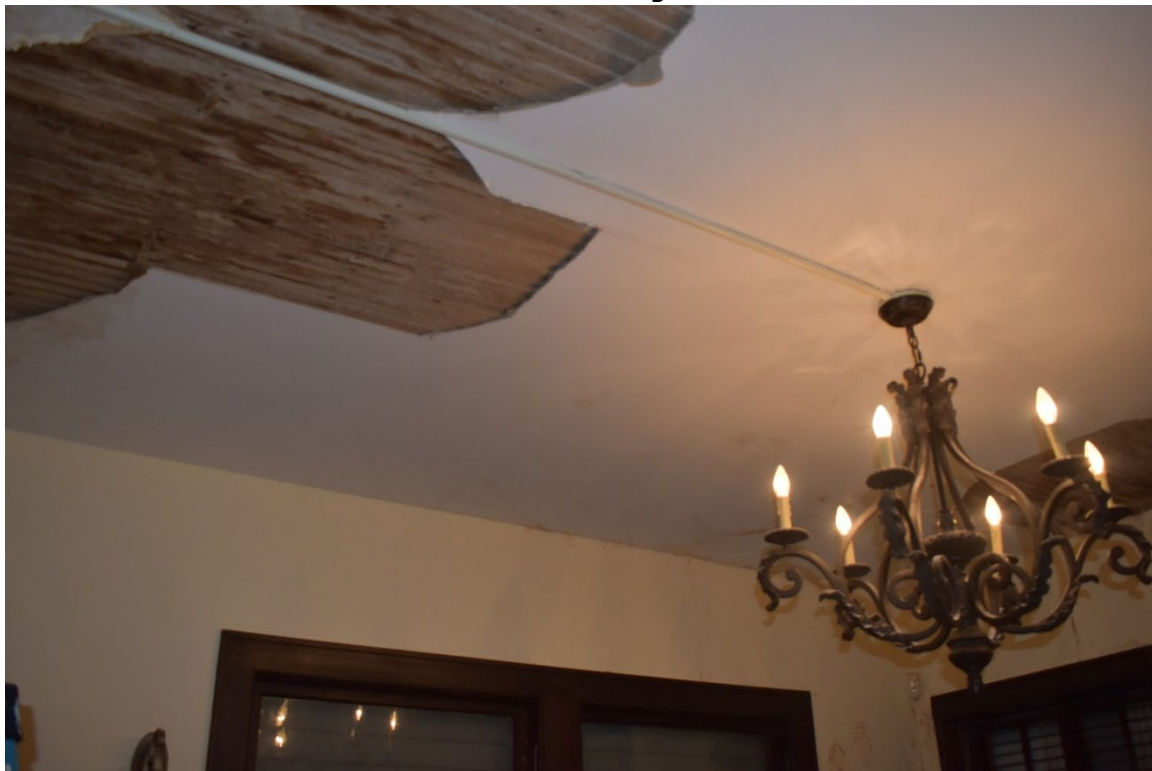
View of damaged ceiling
