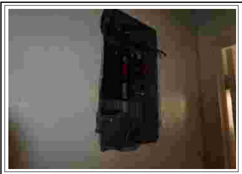
UNIT 1 - ELECTRIC BOX
