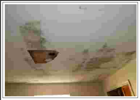
UNIT 1 - WATER DAMAGE
