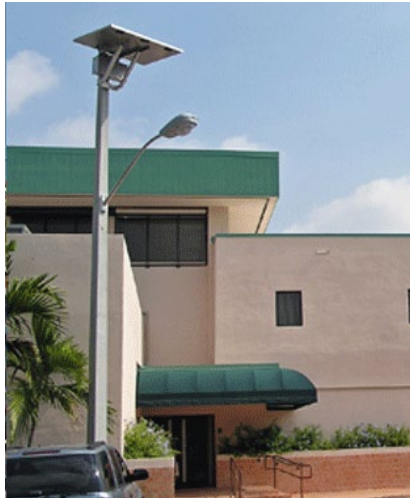
Solar Street Lighting as existing
