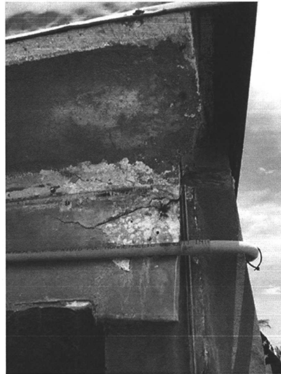
Damaged Walls & Tie-beam
